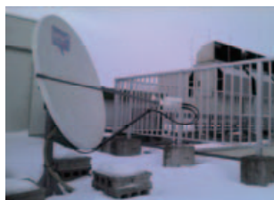
Fig1. Antenna for Satellite IP Network.
